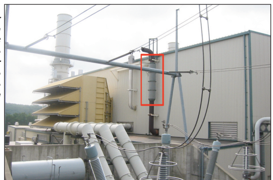
Figure 2. Hogger vent with new IAC lined-pipe silencer on one of three existing units.
