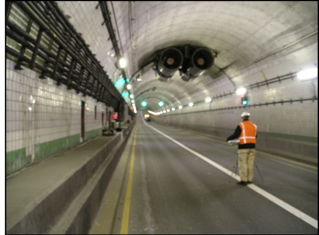
Photo 4. Jet Fan 8 Noise Measurements (Site 4)
